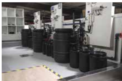
Control equipment that supplies liquid minerals to the plants.
